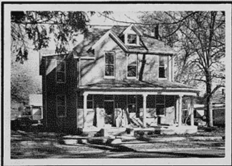
House at 216 Washington Avenue being rehabilitated for the offices of the City's Housing Rehabilitation Services program.
