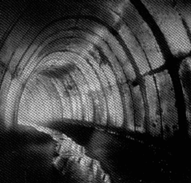
Holland-Tunnel-like is this Evansville sewer, part of the city's excellent sanitation system.
